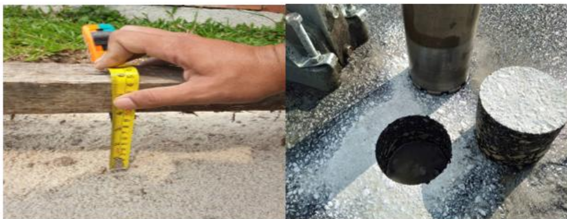
Fig.2. (a) preparation of the concrete slab with 0.1m in-depth, (b) pavement coring procedure
