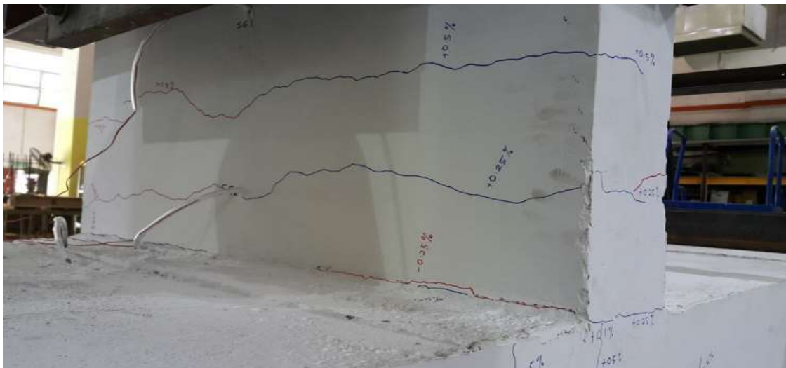
Fig.13. Cracks at wall-slab joint from rear view
