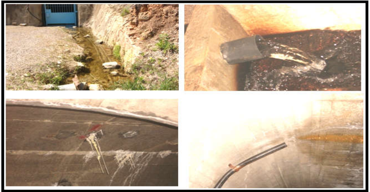
Fig.7. Leaks in the banks of the Gargar dam (Source: Benfetta 2008)
