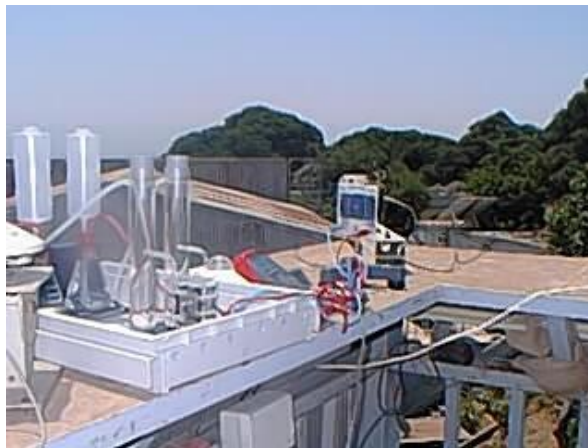
Fig.4. Installation of the production of solar hydrogen in the CDER
