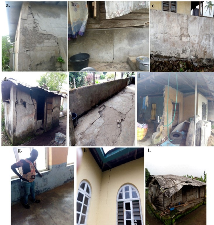
Fig. 4. Photographs taken in 2018 (19 and 18 years after the 1999/2000 eruptions) showing the destruction caused on houses by the 1999/2000 earthquakes from MC in the following localities within Buea Municipality: a-b. cracked wall and foundation in Great Soppo; c-e. old poorly maintained residential buildings in Buea Town with cracked walls and floor; f. partially destroyed inhabited house at Poto-poto quarters in Bokwango; g-h. cracks on walls in buildings at Sasse college; and i. dilapidated wooden house in Tole village
