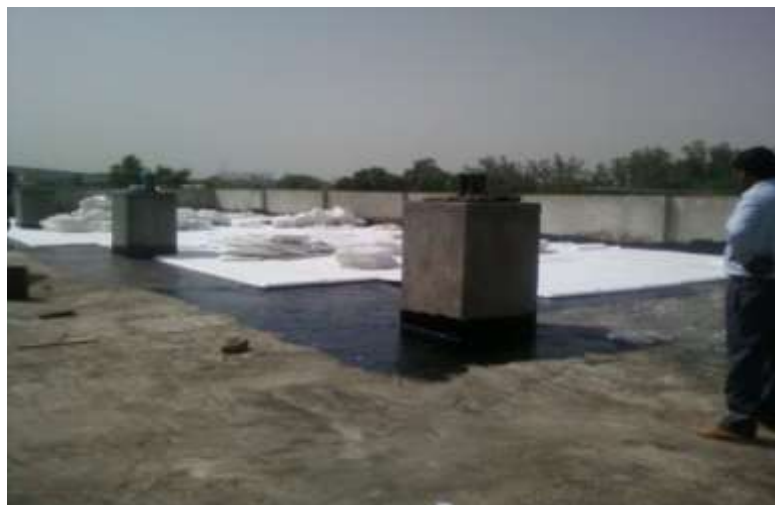
Fig. 12. The insulated EPS sheets are laid on the terrace over a bituminous coat.
