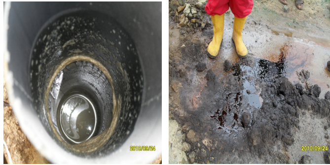
Fig. 8: Top view of exploratory borehole Fig. 9: Oil seepage hotspot near exploratory well
