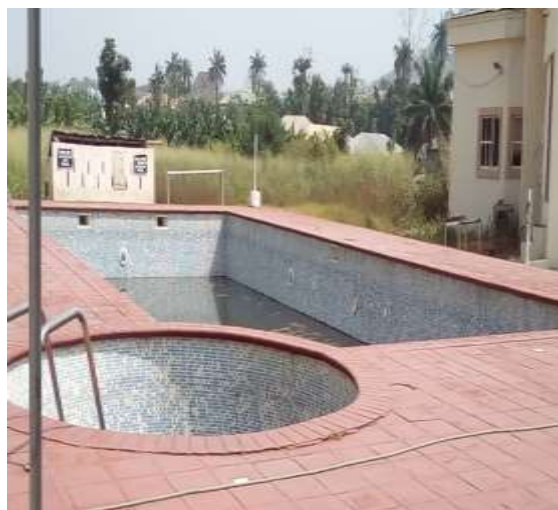
Plate 5. Fountain Hotel Swimming Pool In Bad Condition
