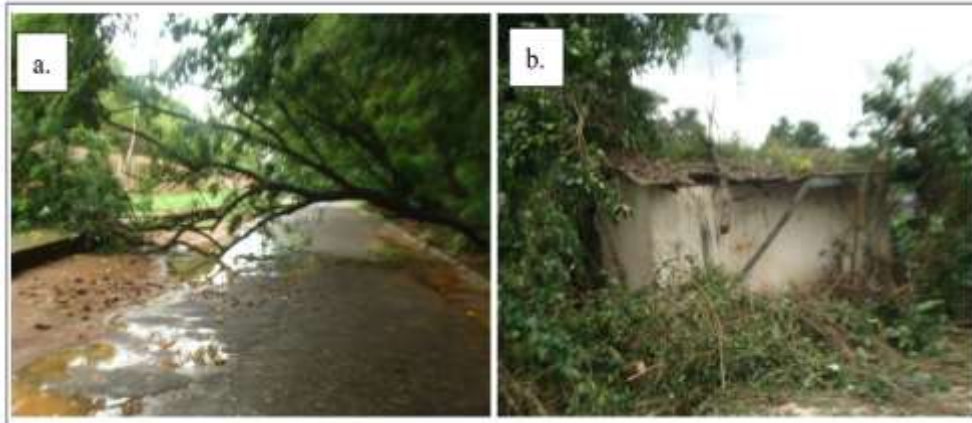
Fig 1: Hazard avenue tree failures leading to A) road obstruction and B) building damage in the university environment (Source: BMC, 2017).
