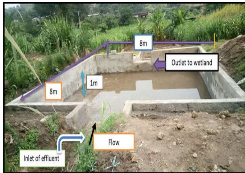
Fig 1: A Constructed sedimentation pond.
