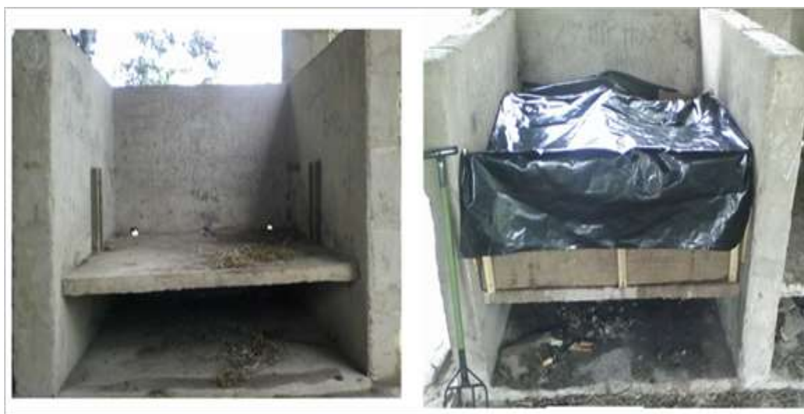
Fig 1: Typical appearance of composting bins
