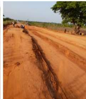
Fig 2b. Longitudinal Cracks
