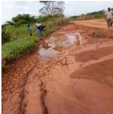
Fig 2a. Alligator Cracking and Edge subsidence
