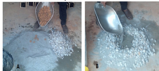
Fig 2: Showing (a) the mixing of concrete constituent (b) mixing of all constituent with water to form concrete
