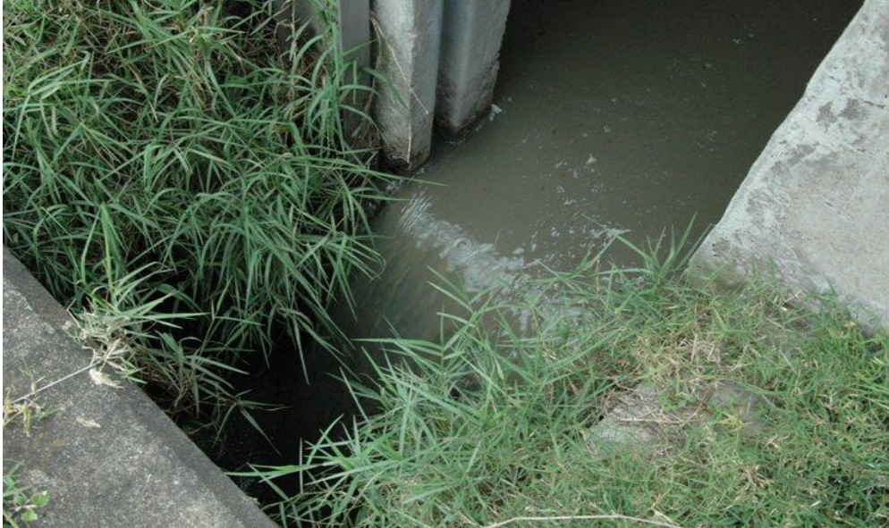
Plate 13: Sewage and storm water draining into Lake Nakuru
