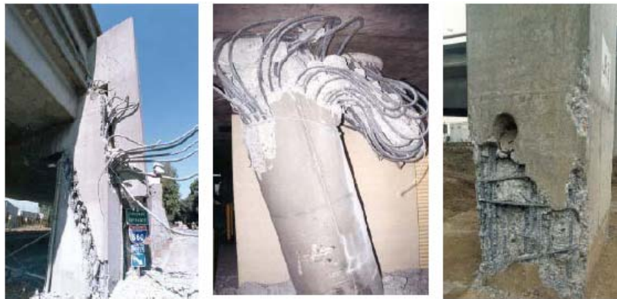
Shear failure mechanism Formation of plastic hinge Insufficient development length Figure 2. Common failures in columns that occurred in 1989 during the Loma Prieta Earthquake
