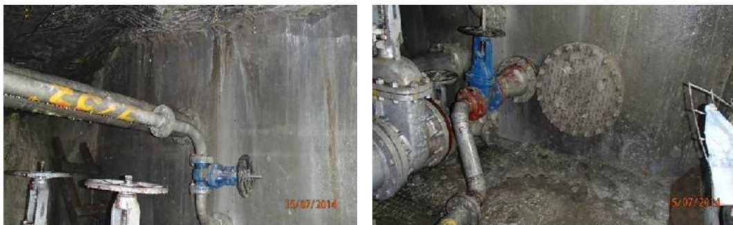
Figure 1. Leakage of an underground water tanks (Source: Bulyanhulu Gold Mine)
