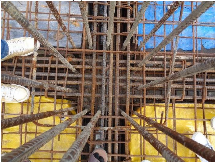
Figure 8: Rebar cluster in a joint, where bottom reinforcements were uncut
