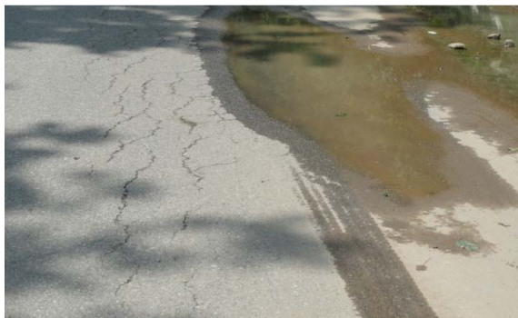
(a) Water Logging Near Chainage km 233.800
