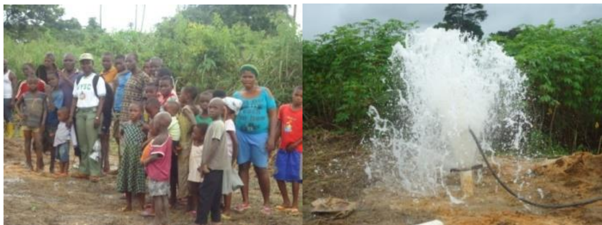
Fig 18: Corps Member Okoye Sheila Chizoba (AK/12C/0868) and the people of Ikot Enini , Edemaya during the drilling process.
