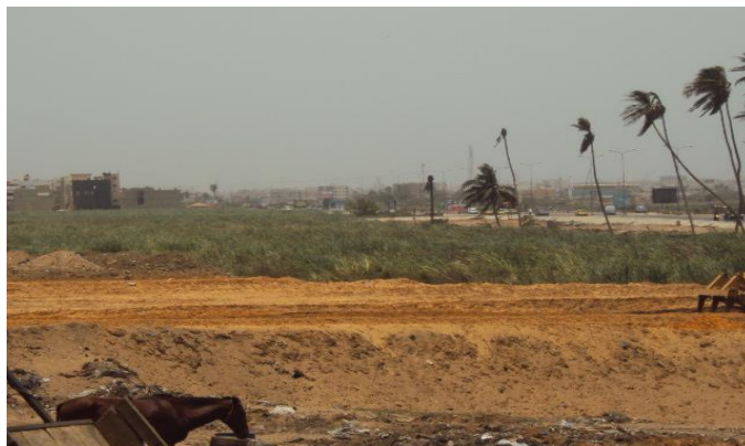
Figure 11: Backfilling carried out in 2015 in the Niaye area of Pikine for the building of the National Wrestling Arena.
