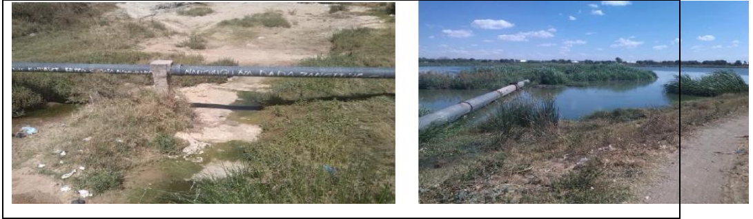
Figure 4: Sewerage pipes in Makole street transporting wastewater to Swaswa WSP
