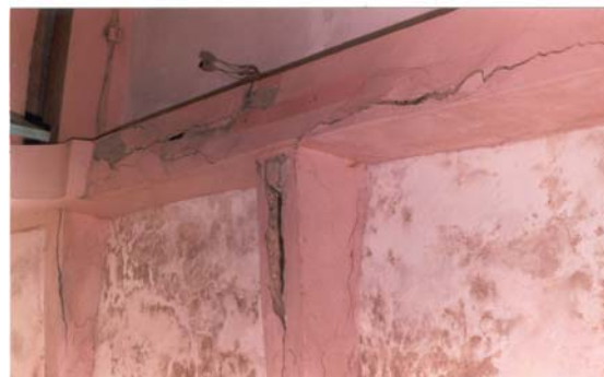
Fig. 2 Serious Multiple Crack Damage in Building Attributed to Blasting
