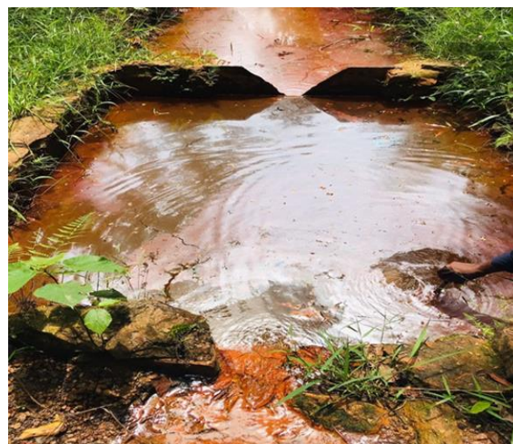
Fig. 1 Conduit Producing Reddish-Brown Effluent Suspected to be AMD
