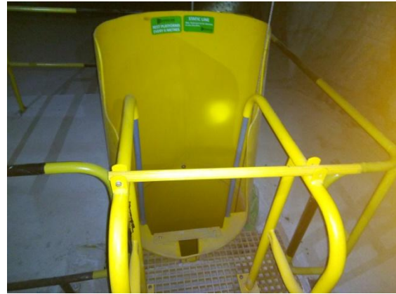
Fig. 5 Safescape Ladder Tube at CGML
