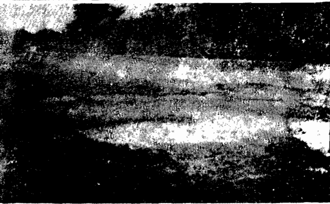
Fig. 5 Evidence of poor pavement condition
