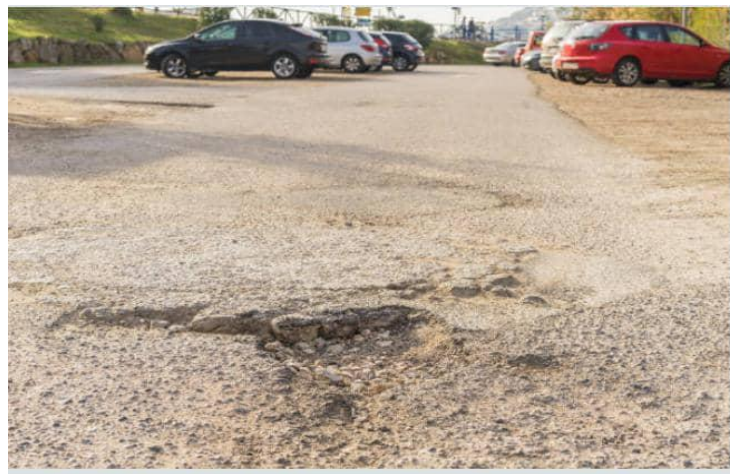
Plate 1: Pothole causing Traffic Obstruction along Felele Road, Lokoja Source: Author’s Fieldwork, 2023
