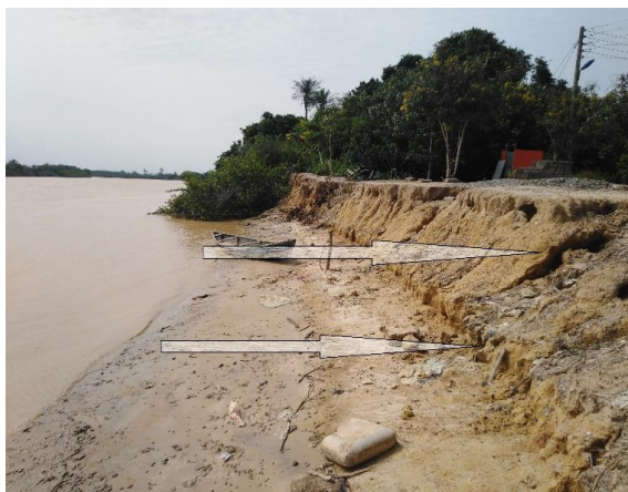
Figure 4a: Riverbank erosion at Krobo Source: Field survey, 2019
