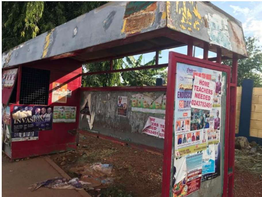
Figure 21: Poorly maintained rest stop at Opoku Ware School
