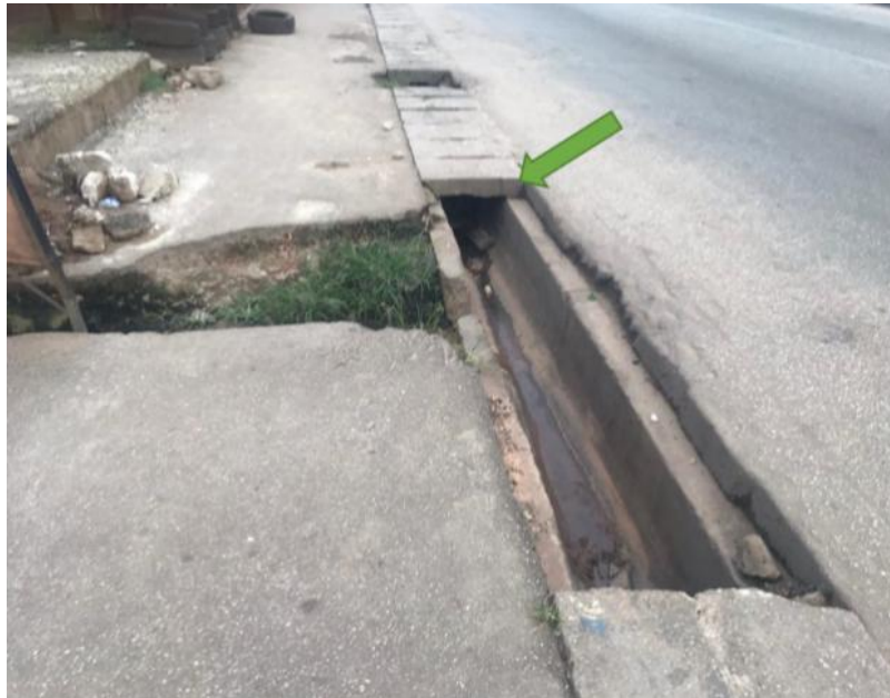
Figure 15: Partly covered drain at Suame
