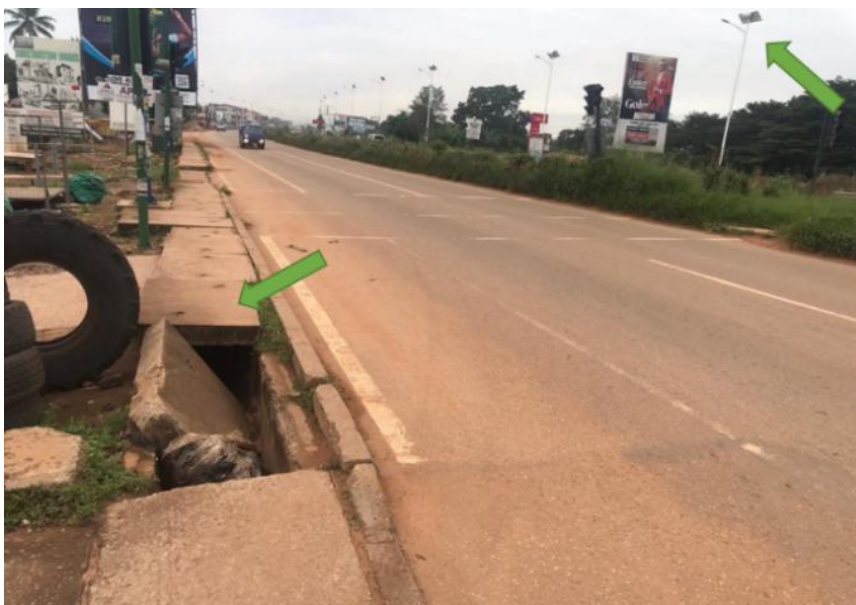
Figure 16: Uncovered drain and street lighting along the Adum-Tanosu road
