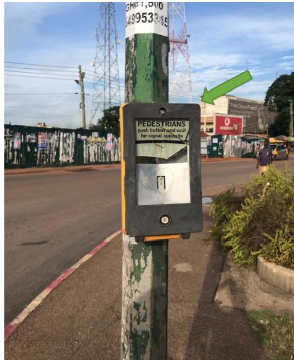
Figure 18: Poorly maintained traffic light
