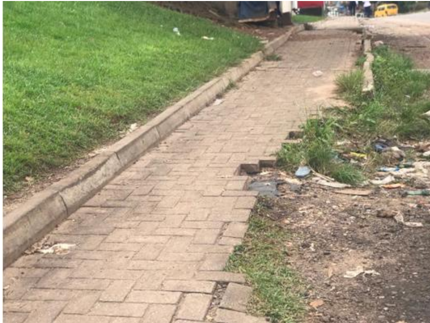
Figure 5: Maintenance challenges with side-walk at Suame
