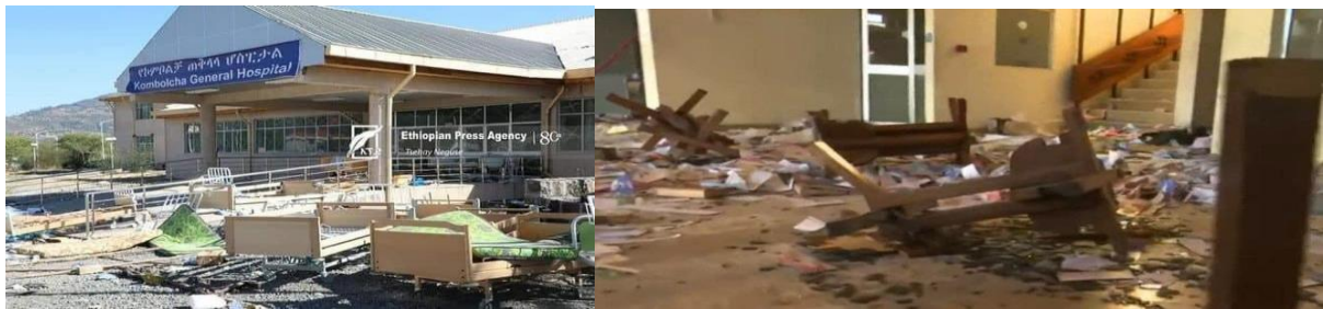
Figure.12. the damaged Hospital at Kombolcha-Amhara-Ethiopia
