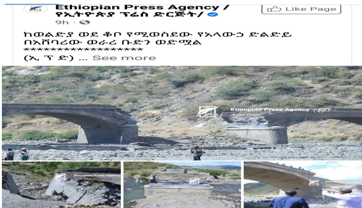
Figure.17. Damaged Infrastructure by TPLF @Amhara Region
