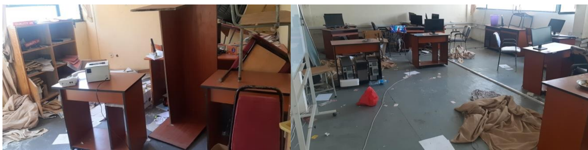
d. Damaged Wollo University (KioT) by TPLF
