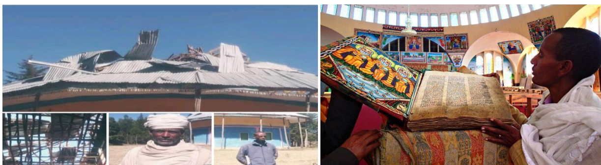
Figure.a. Damaged Church by TPLF in Mekite-Amhara
