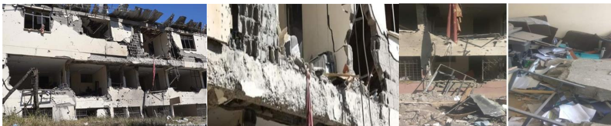
e. Damaged Wollo University (Dessie Campus) by TPLF
