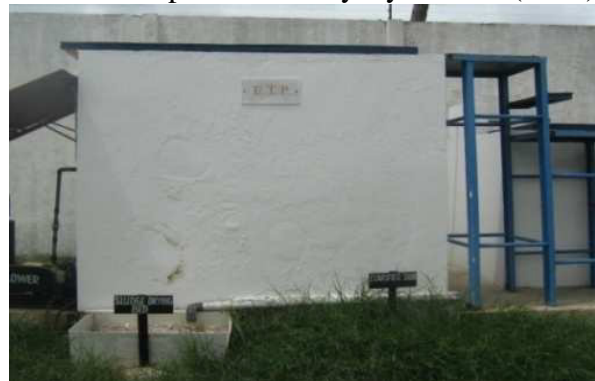
Plate 1a Fluidized Aerobic Bio Reactor (FAB)
