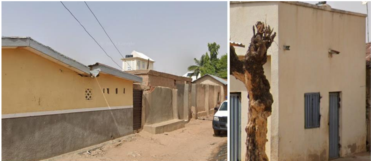
Fig. 11 Buildings devoid of structural cracks in the stable zones around FCE, Gombe
