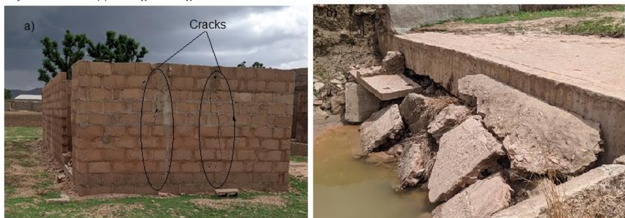
Fig 8 (a) Cracking walls of a new building in the unstable zones, (b) A collapsed bridge founded on the clays of Kanawa.
