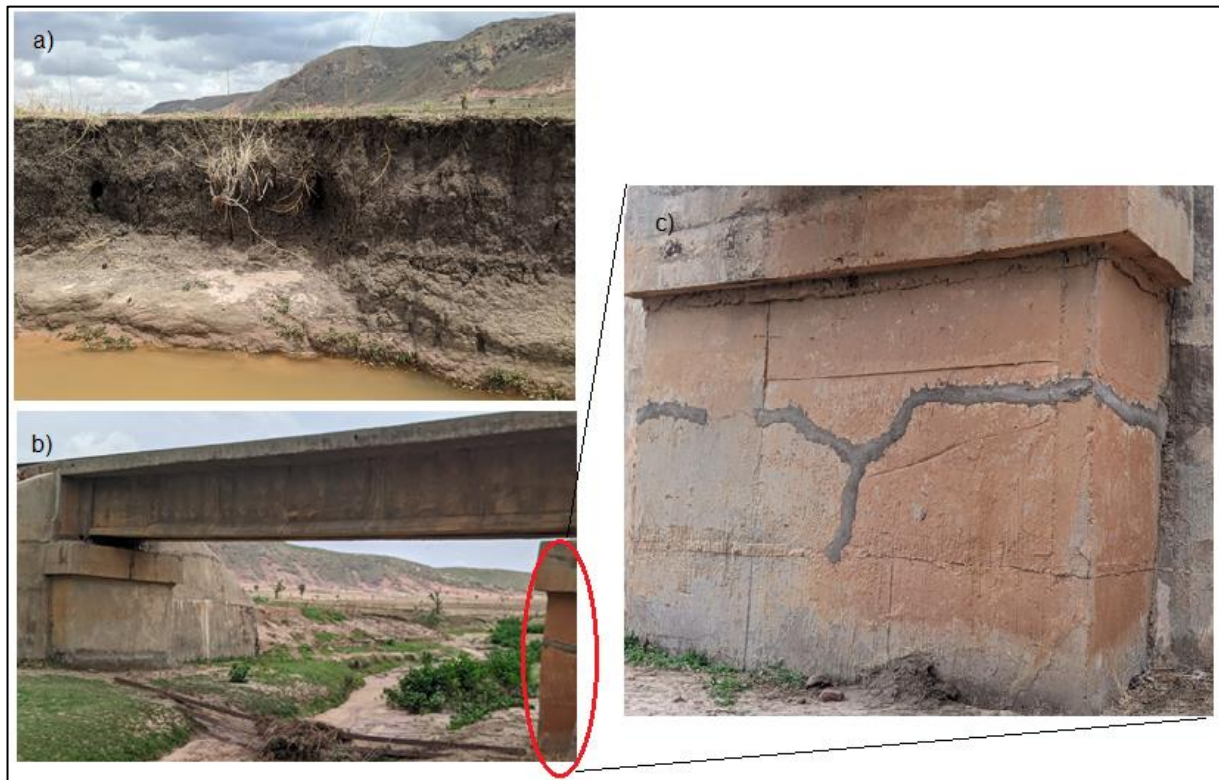
Fig 7 (a) Weak clays of Kanawa member which underlies the unstable zones, (b) A failing bridge founded on the clays of Kanawa, (c) Enlarged bridge abutment with massive cracks
