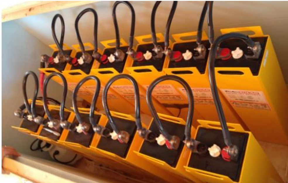
Figure 3: Battery bank (Franklin, 2017).
