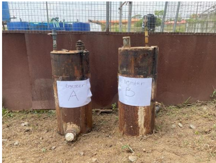
Plate 1. The floating drum digesters
