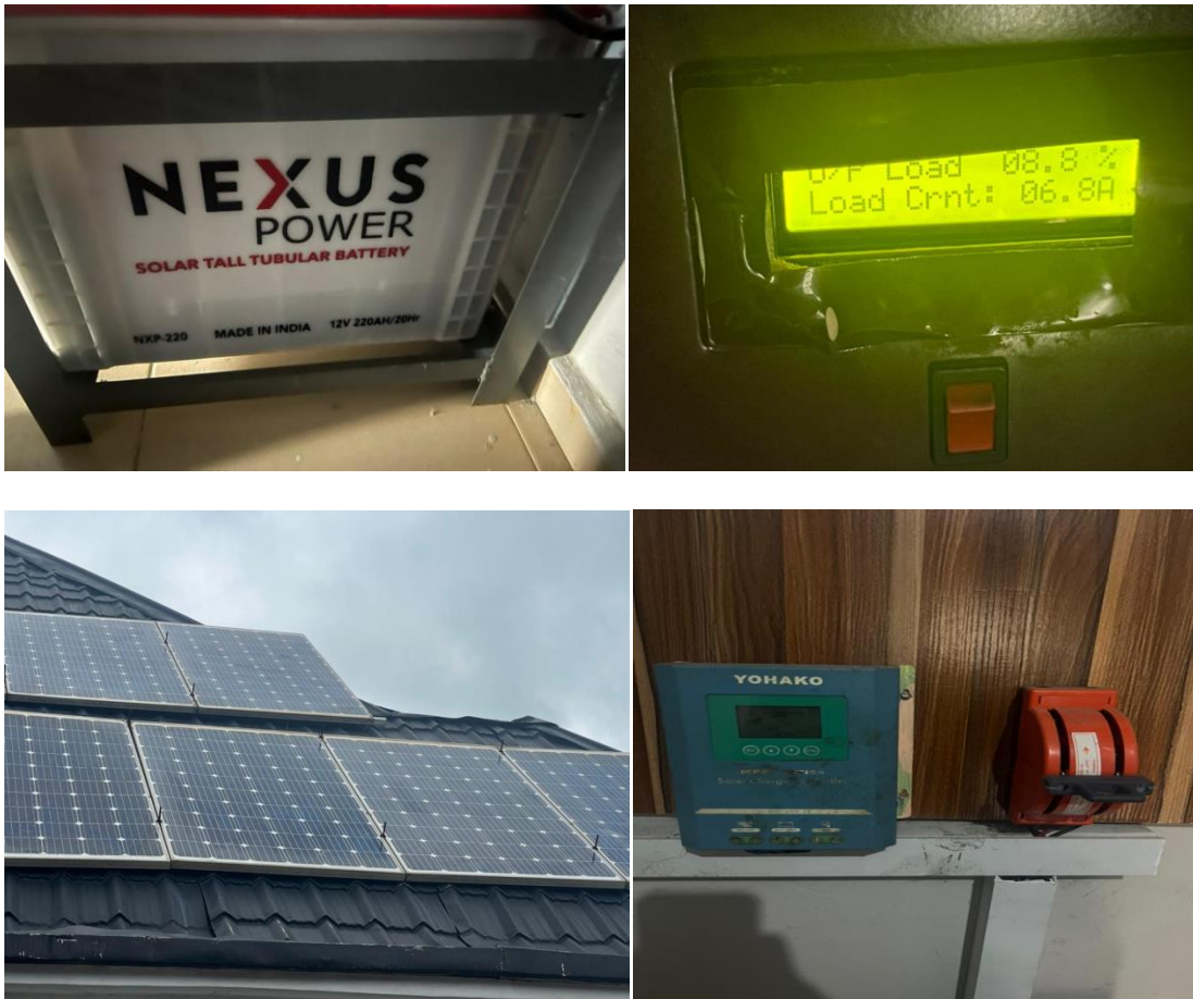
Figure 2: Pictorial view of the system arrangement (a) Power Battery (b) Inverter System (c) Solar PV array (d) Charge controller and Service box
