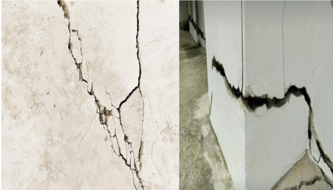
Figure 1: A typical failed building with cracks down to the foundation in the study area.
