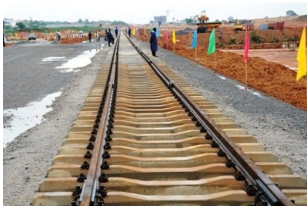
Figure 7. A View of the Abuja-Kaduna Rail Line Project Source: http://www.railway-technology.com/projects/abuja-kaduna-rail-line/ (Retrieved May 2024).
