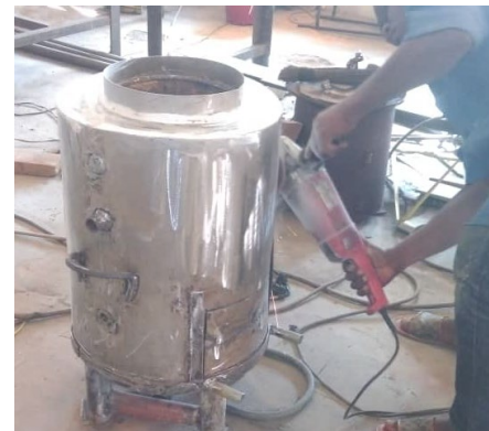
Plate 3f: Furnace shell
