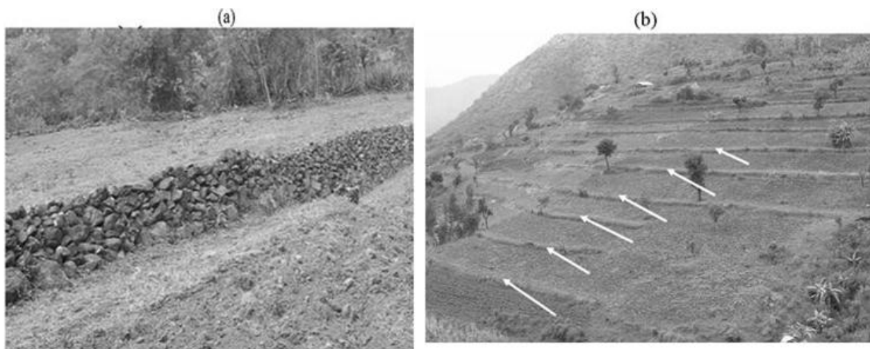
Figure 4. Stone bunds in lower watershed; (a) newly built stone bund; (b) series of stabilized stone bunds with grass, six years after construction.
