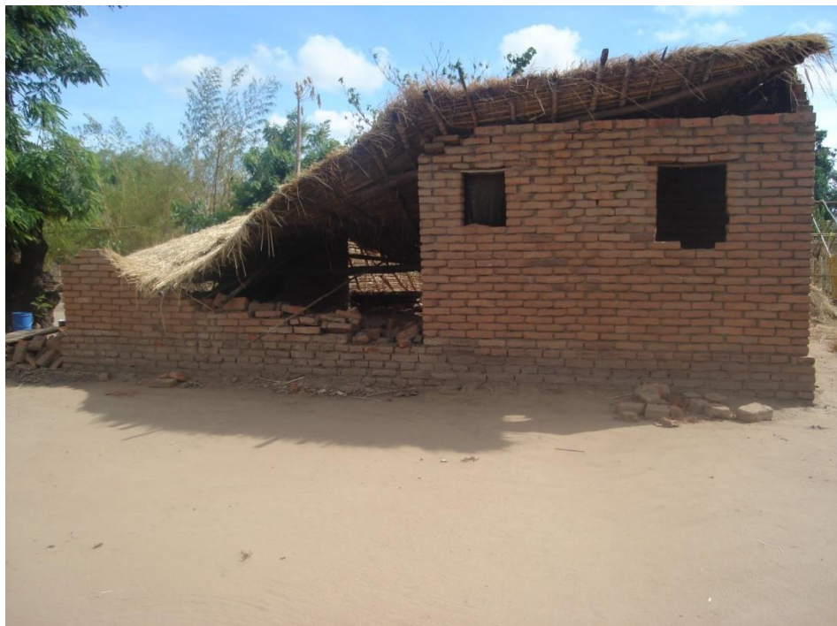
Figure 7. One of the affected houses in Karonga Town-(Picture by Kushe, 2015).
