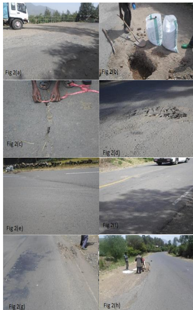
Fig. 2(a): Photograph image showing pavement distress of a road segment between Kemissie and Dessie; Fig.2(b): Sample -I collection from pavement dislodgement; Fig.2(c): Sample-II collection from transverse crack; Fig. 2(d): Sample-III collection from patched pavement; Fig. 2(e): Sample-IV collection from non-uniform road surface; Fig. 2(f): Sample-V collection from distorted road surface; Fig. 2(g): Sample-VI collection from sheared road surface; Fig.2(h): Sample-VII collection from potholed pavement.
