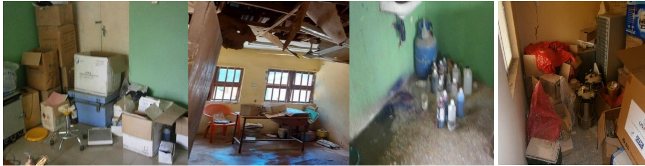
Fig 7: A store without cabinets, leaking ceiling of a store, and consumables/supplies on the floor of a store in one of the selected health facilities, Sokoto State, Nigeria
