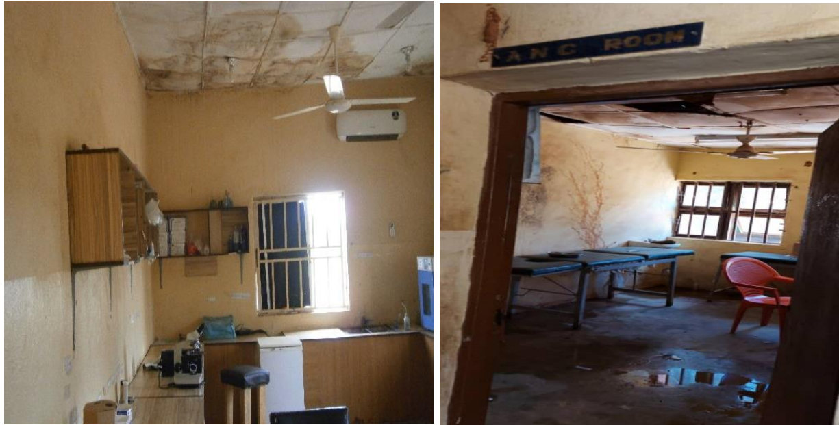
Fig 2: Laboratory without benches and with dilapidated equipment and leaking roof in selected health facilities, Sokoto State, Nigeria
