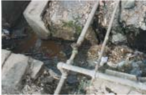
Plate 3: An Open Drainage And Pipes, Which Are No Longer Useful
