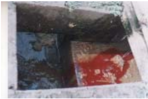
Plate 4: Manure mixed With Blood flowing into an open Drainage from the main slaughter hall
