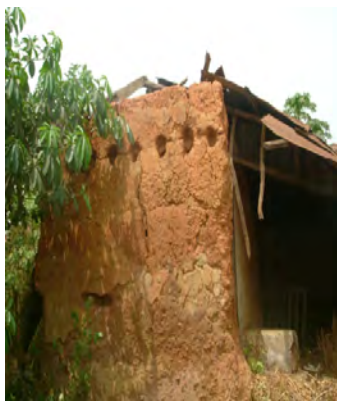
Lejoka's dilapidated Palace
