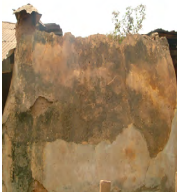
Odole's dilapidated wall
