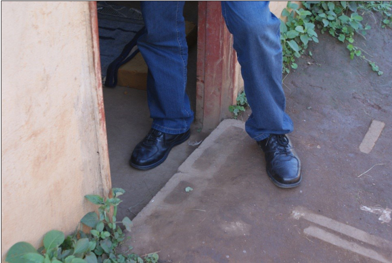
Figure 7: Example of poor substructure in low-income houses
