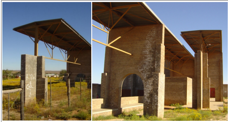
Figure 9: No maintenance on the cement brick-constructed Steinkopf Community Centre in the Northern Cape Province, South Africa
