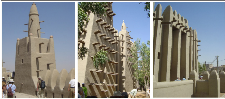
Figure 15: The restored rooftop with minarets, tower and facade of the Great Mosque of Mopti
