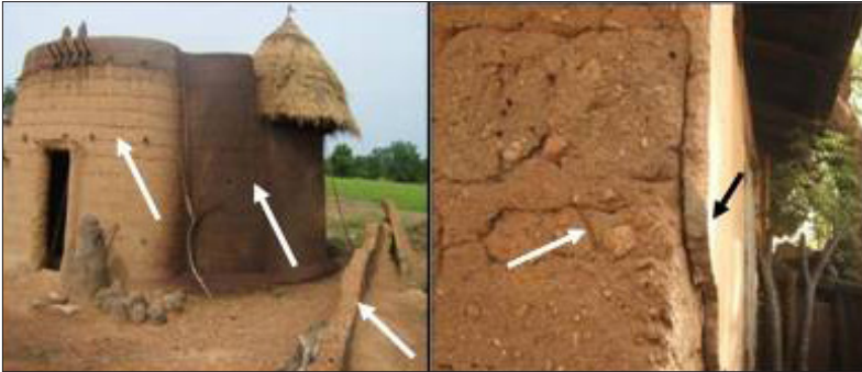
Figure 15: Traditional earthen buildings deterioration due to water penetration showing the urgent need for wall coatings in Benin
