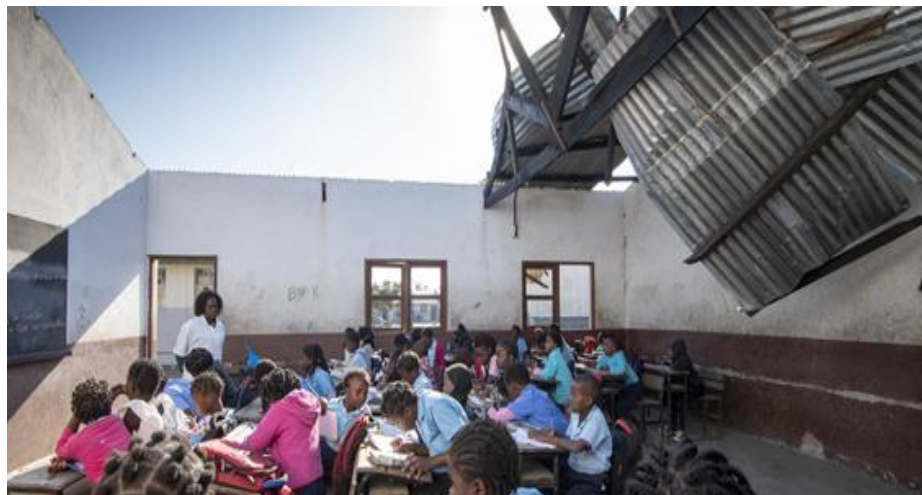
Figure 2: - Escola 25 de Junho, in Beira, Mozambique, damaged during Cyclone Idai
