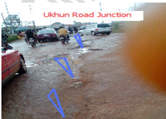
Figure 9: Picture taken at the Ukhun Road Junction opposite General Hospital, Ekpoma. Note the arrows indicating parts of the road excavated without sealing it up properly.
