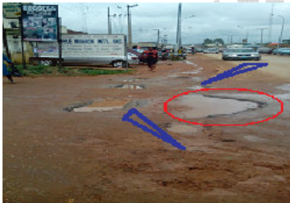
Figure 4: Picture taken at the Oguamelen Street Junction near UDA Microfinance Bank, Ekpoma. Observe the blue arrows indicating part of the road excavated without sealing it up properly, and the encircled part where further degradation has begun
