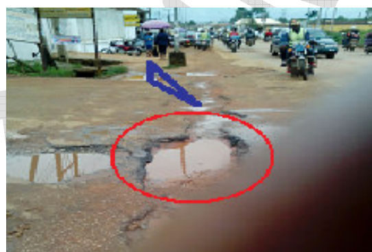
Figure 3: Picture taken at the Afua Street Junction near Fin Bank Plc, Ekpoma. Observe the blue arrow indicating part of the road excavated without sealing it up properly, and the encircled part where further degradation has begun.
