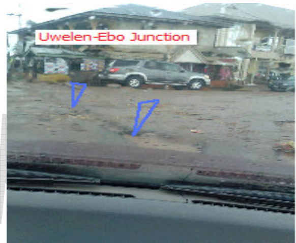
Figure 10: Picture taken on a rainy day from the interior of a car at the Uwelen-Ebo Junction opposite Eko Bank Plc, Ekpoma. Note the arrows indicating part of the road excavated without sealing it up properly.
