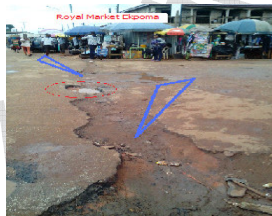
Figure 7: Picture taken at the Aburime Street Junction near Royal Market, Ekpoma. Note the arrows indicating part of the roads excavated without sealing it up properly. Observe also the encircled part of the right side where further degradation has begun.
