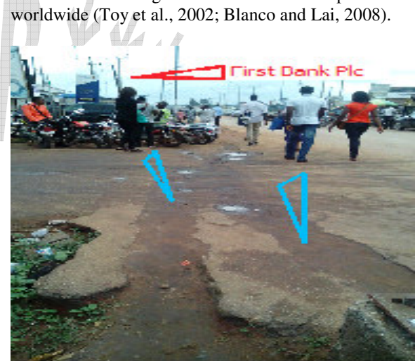
Figure 6: Picture taken at the Isidahome Street Junction near First Bank Plc, Ekpoma (see RED arrow pointing towards the bank). Observe also the arrows indicating part of the road excavated without sealing it up properly.
