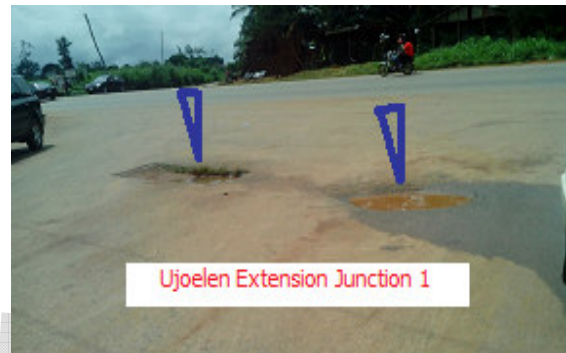
Figure 1: Picture taken at the Ujoelen Extension Junction (1) directly opposite G2 Road, Ekpoma with the Benin-Auchi Express way running across. Note the blue arrows indicating parts of the road excavated without sealing them up properly.
