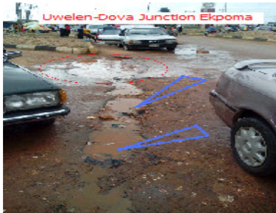
Figure 8: Picture taken at the Uwelen-Dova Junction opposite Royal Market Square, Ekpoma. Note the arrows indicating the parts of the roads excavated without sealing it up properly. Observe also the encircled portion where severe degradation has begun.
