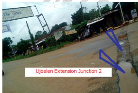
Figure 2: Picture taken at the Ujoelen Extension Junction (2) directly opposite Ujoelen Road, Ekpoma. Note the BLUE arrows indicating part of the road excavated without sealing it up properly.
